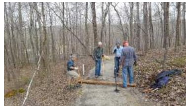
Positioning water bars on our eight miles of hiking trails is no easy task. At a trails work day on March 30, Don Williams, Tim Bigelow, Les Hook, and Jim Given discuss the best way to position the cedar log before securing it.
